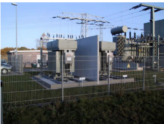
Figure 3: 20kV twin busbar distribution, RCC Ground Fault Neutralizer, with solid-core arc suppression coils (courtesy WEMAG Vattenfall Europe)
