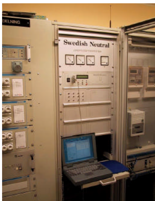
Figure 7: First RCC Ground Fault Neutralizers in Sweden, 1992
