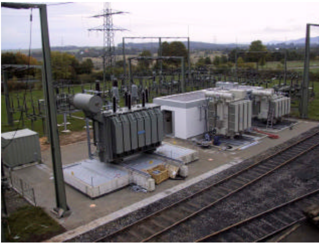
Figure 2: 110kV / 16.7Hz, German national railway transmission system, RCC Ground Fault Neutralizer, plant overview (courtesy Deutsche Bahn)
