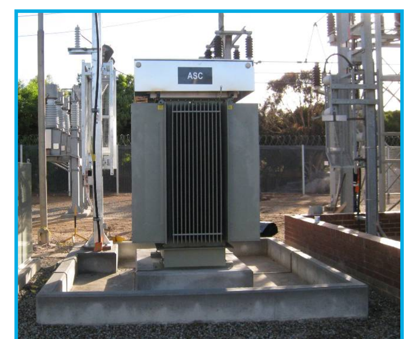
Arc Suppression Coil (ASC)
