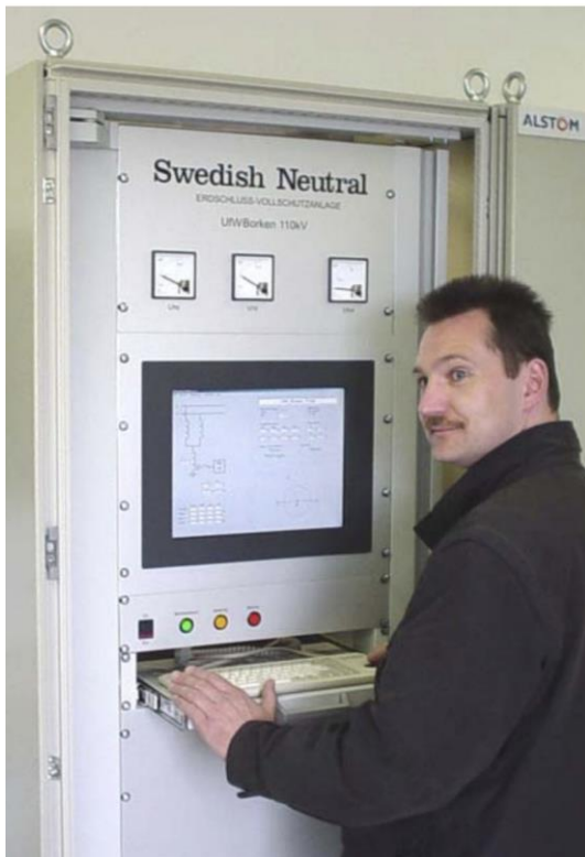
Figure 1 Modern Neutral treatment with Ground Fault Neutralizer, German Railway 110kV transmission system (courtesy Deutsche Bahn)
