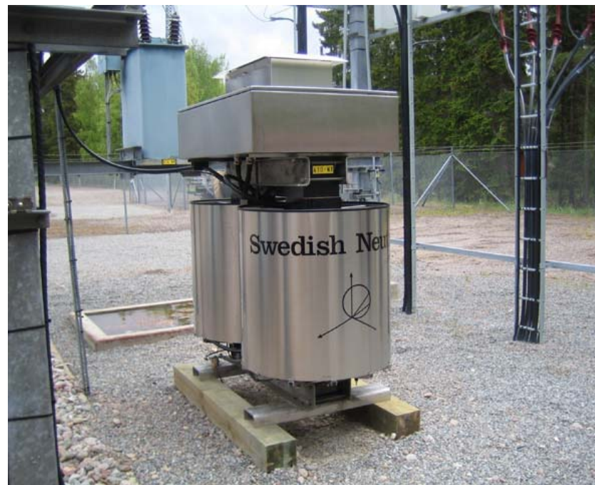
Figure 3: Modern dry-type arc suppression coil for distribution networks
