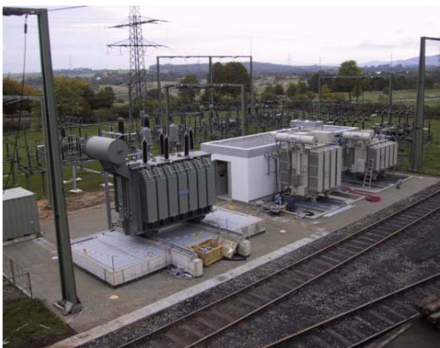
Figure 2: 110kV German railway transmission system, RCC Ground Fault Neutralizer, plant overview (courtesy Deutsche Bahn)
